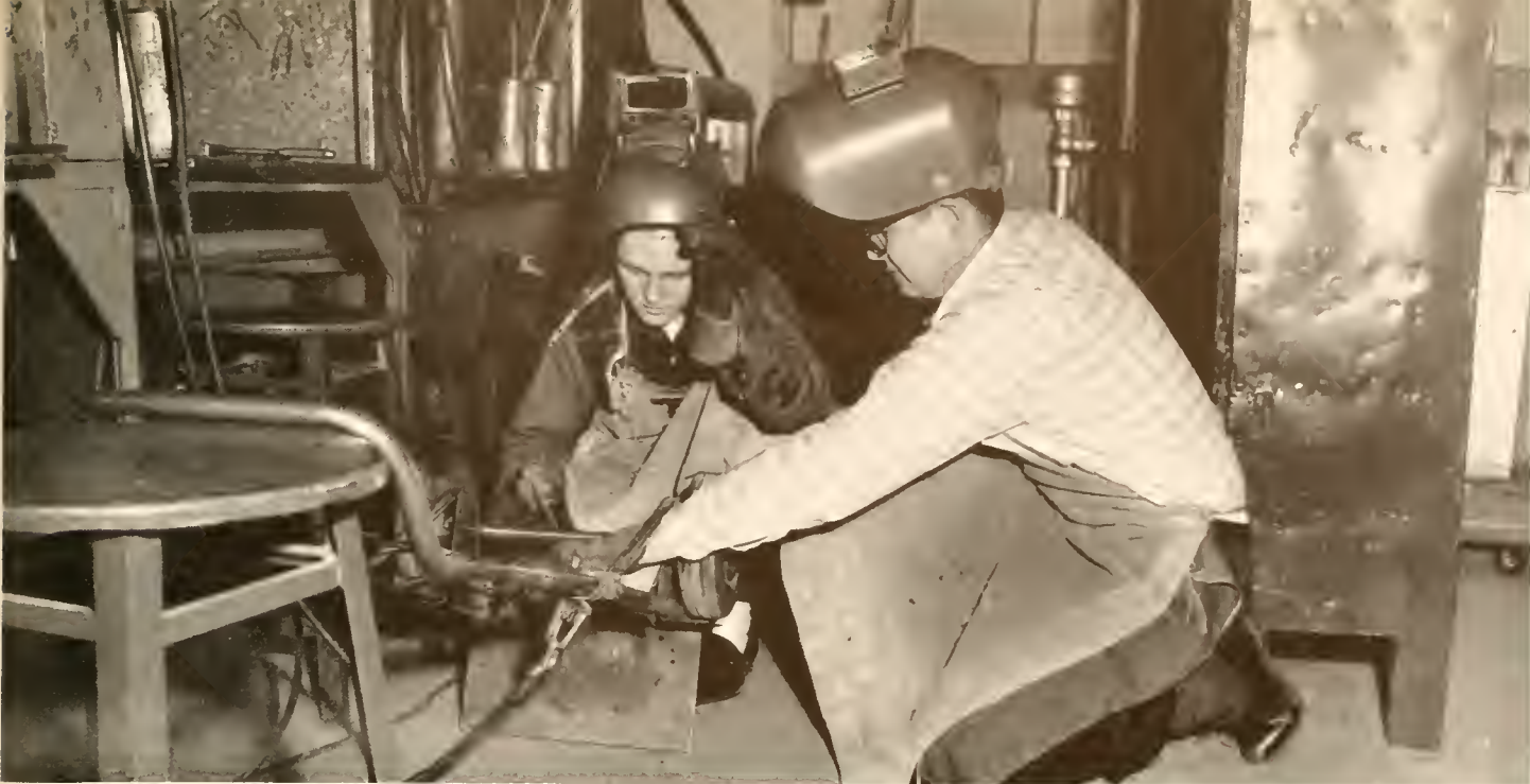
These welders (not spacemen), Dick Johnson and Ken Lowden, examine a piece of metal in shop class.
